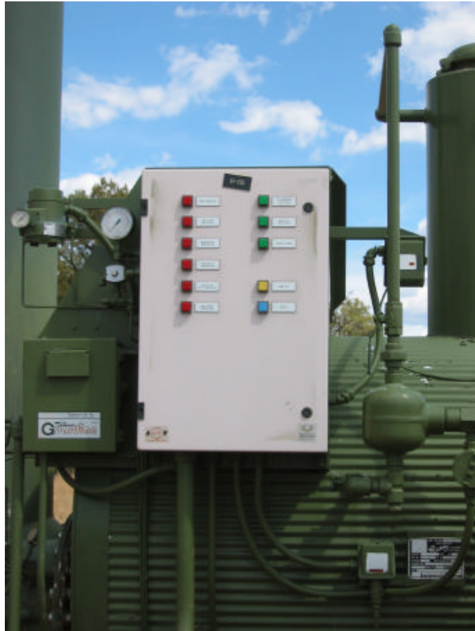
Figure 6: Alarm Panel on the CO 2 Heating Unit, Allison Unit
