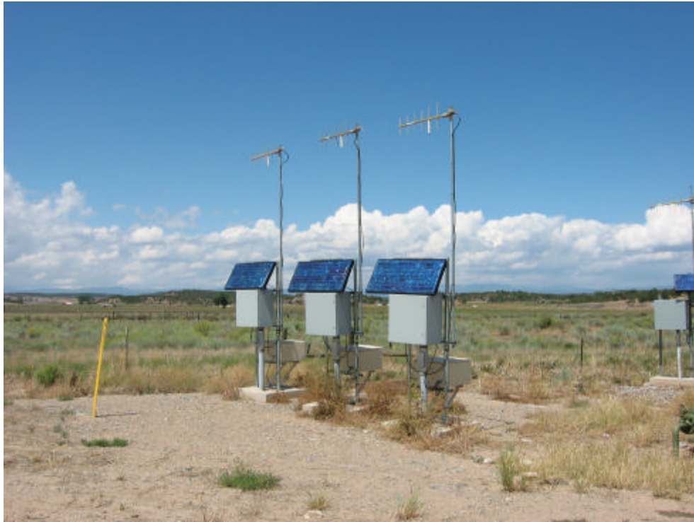
Figure 19: Onsite Power Source and SCADA Transmission System, Tiffany Injection Wells (three wells)
