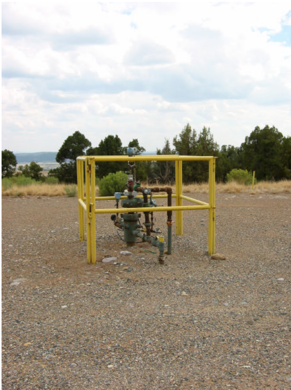
Figure 22: Production Wellhead, Tiffany Unit
