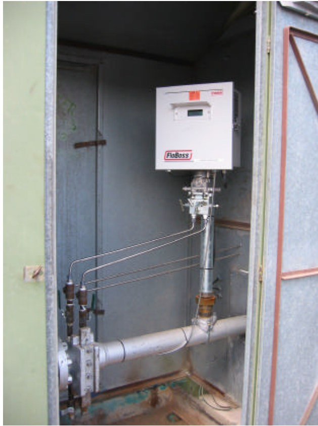
Figure 11: Gas Flow Meter, Allison Unit Production Well
