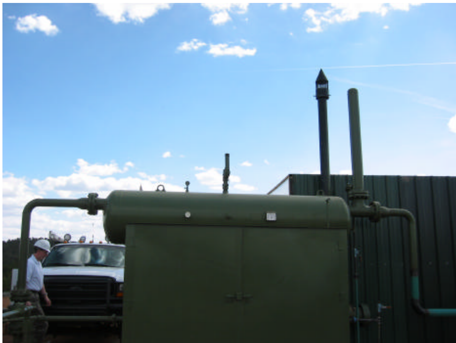
Figure 10: Gas/Water Separator, Allison Unit Production Well
