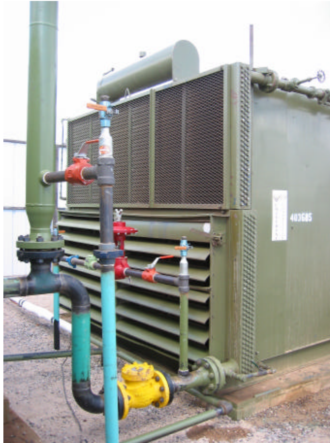
Figure 13: On-Site Compressor, Allison Unit Production Well
